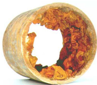
Figure 1: Internal rust collection.
