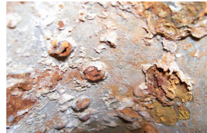
Figure 3: Microbiologically induced corrosion
