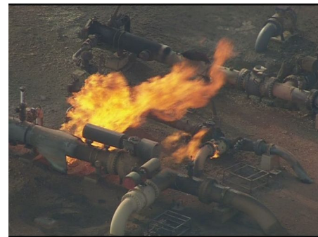
Figure 4: Petroleum pipeline bursting.
