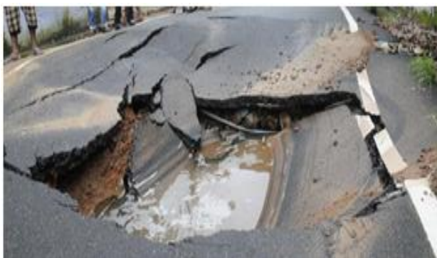
Figure 4: Damage of road due to pipeline burst.
