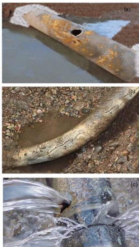
Figure 1: Damages in water pipelines due to corrosion flaws.
